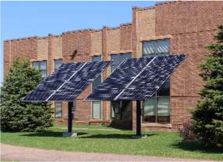
Minnesota Municipal Power Agency 5 kW Hometown Solar Shakopee, MN
